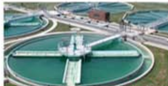
Effluent Treatment Plant (1.5 MLD)
