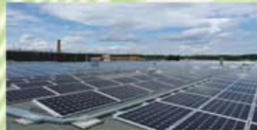
Roof Top Solar Power Plant
