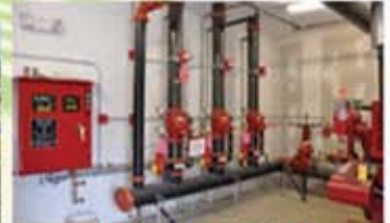
Hydrant Pump Systems
